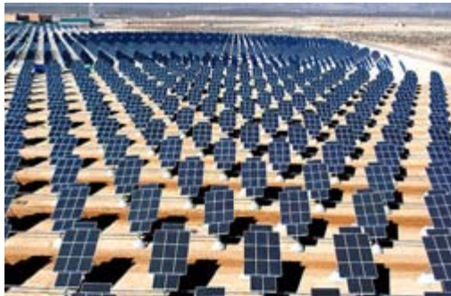
At Nellis Air Force Base, 70,000 solar arrays generate 15 megawatts of power.
